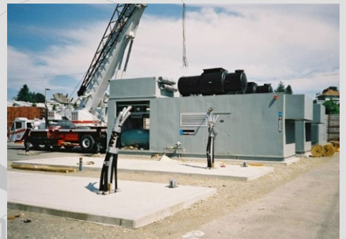
One of the new power generators at the Vancouver International Airport
